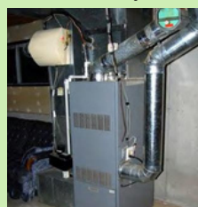
Whole-house forced-air ventilation system
